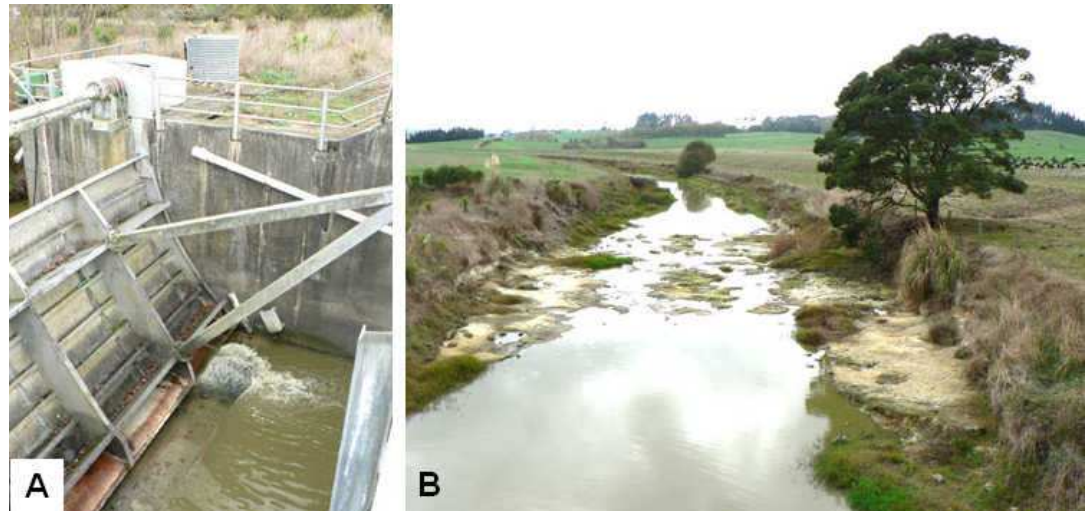
Figure 2: A) The control gate in the closed position on the Pungarehu canal. B) The Pungarehu canal flow with the control gate closed (Photos: M. Gibbs, 14 April 2008).
