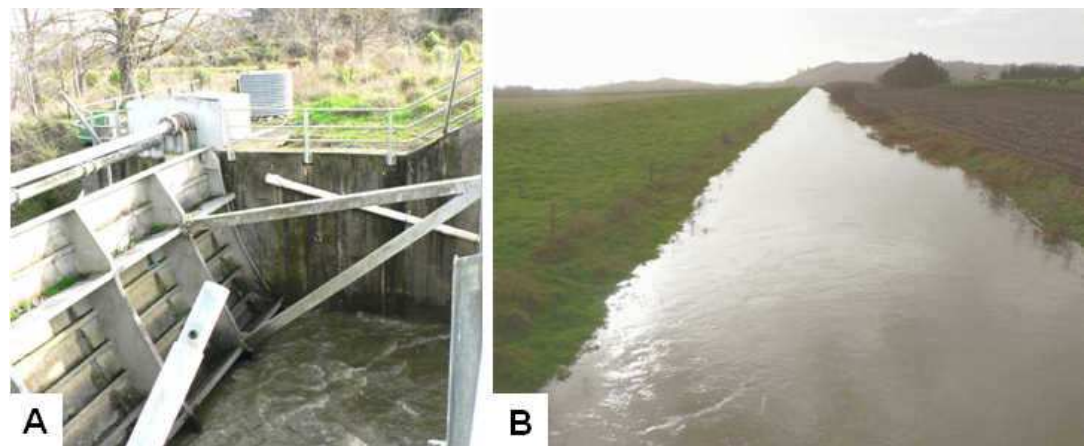
Figure 3: A) The control gate in the open position on the Pungarehu canal. B) The Pungarehu canal flow with the control gate open (Photos: M. Gibbs, 23 June 2008).
