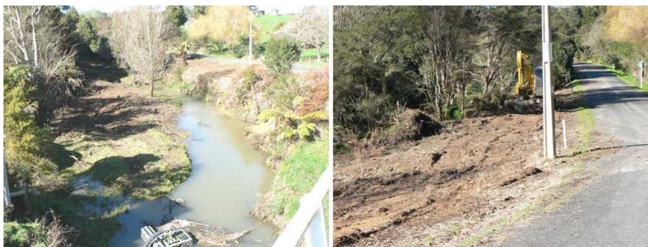
Figure 15: In-stream and bank earthworks in the upper Waerenga Stream catchment, 24 July 2008 (Photos: M. Gibbs).
